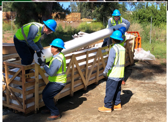
Chinese carpenters construct a distinctive curved roof on a small streamside pavilion. Inset: Materials shipped from China are unpacked.
